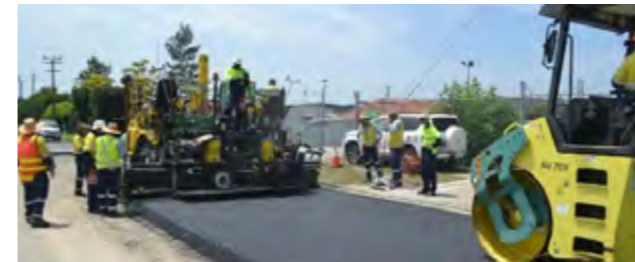
Application of Enrobés à Module Elevé Class 2 (EME2) technology in Brisbane City Council.
