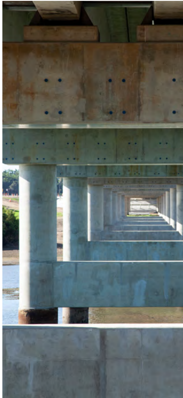
The underside of a new reinforced concrete bridge across the Pioneer River at Mackay, Queensland, showing pylons and beams reducing in size. Image Source: IngeBlessas Shutterstock (2024)
