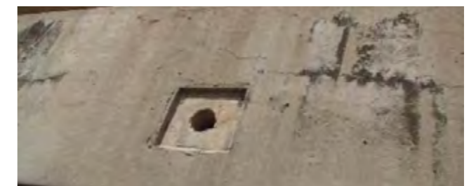
End 1 stress bar broken, Bridge ID 625 (Oct 2016 L2 inspection) Image Source: NACOE (2019)
