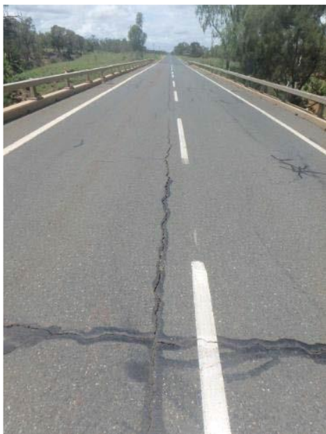
Full length crack running from A1 to A2 down bridge centreline
