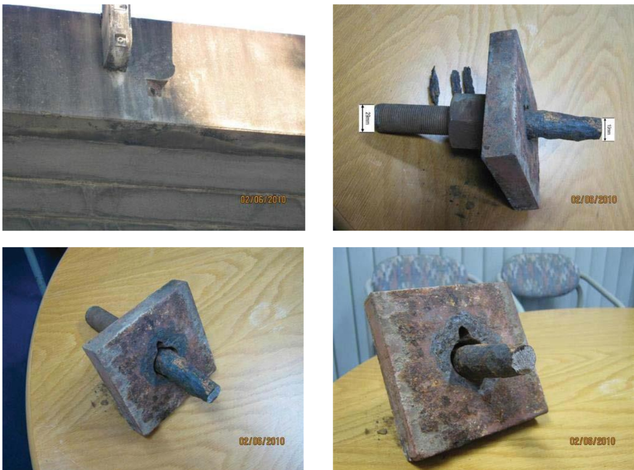
Figure 3.2: Broken sections of TSB on Bridge ID 7330 (Jun 2010 L2 inspection)
