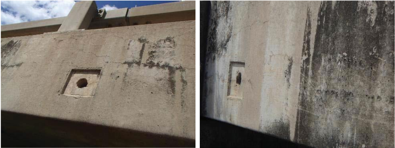
Figure 3.1: End 1 stress bar broken, Bridge ID 625 (Oct 2016 L2 inspection)
