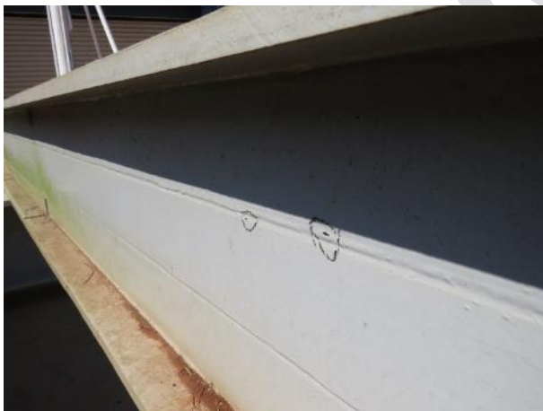
Figure 3.6: Coating defect, holes noted due to air bubbles on painting, Girder 1-6
