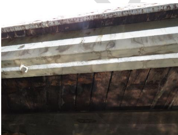
Figure 5.2: Typical water stain along FRP girder
