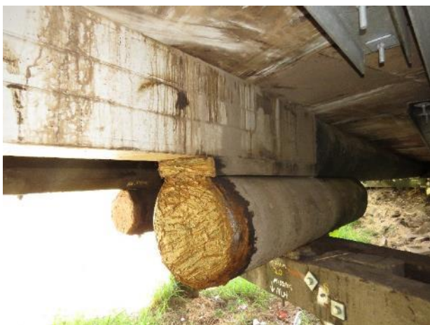
Figure 5.23: View of typical water stain at the FRP girder
