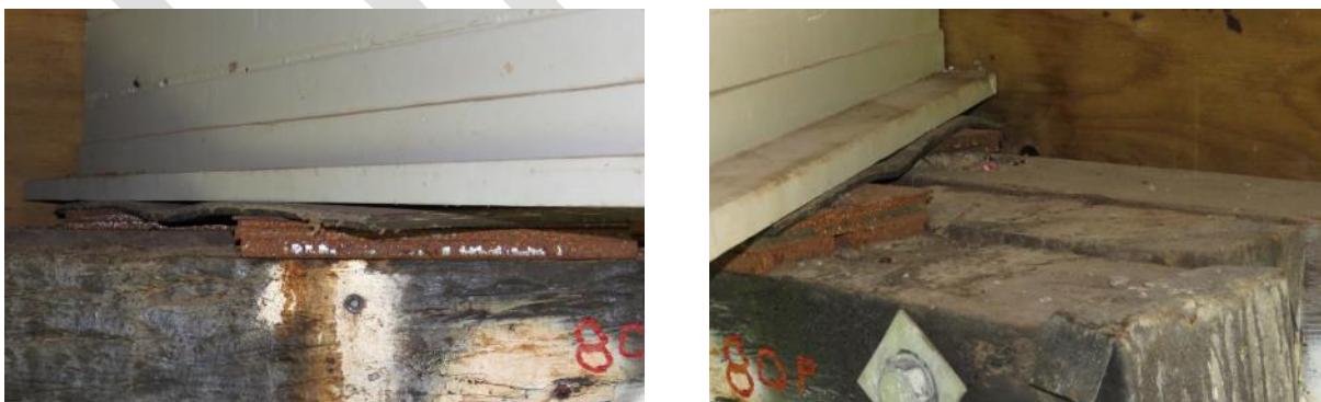
Figure 5.10: Bulging of rubber pads at bearings
