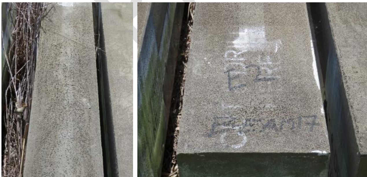
Figure 3.23: Pitting defects on the top surface of girder 17
