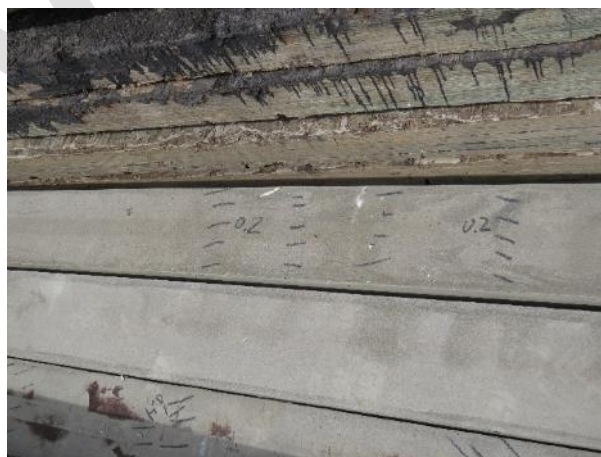
Figure 3.28: Cracking on top of girder 8 at mid-span
