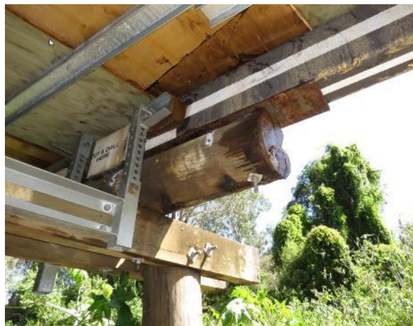
Figure 5.17: Corroded steel plate between FRP girder (S3-G1) and corbel (P2-COR1)
