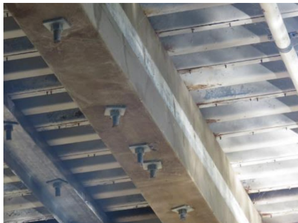
Figure 5.29: Corrosion of steel trough in contact with the FRP girder
