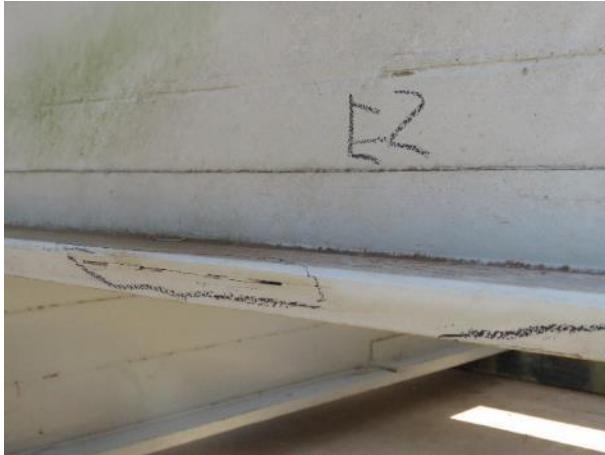
Figure 3.4: Typical delamination noted at bottom flange of Girder 1-6
