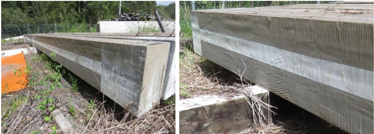
Figure 3.24: Typical deformation of the coating of resin
