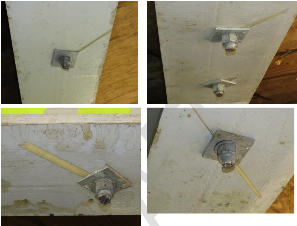
Figure 5.9: Strip of fibre removed at the soffit of girder, close to a bolt connection
