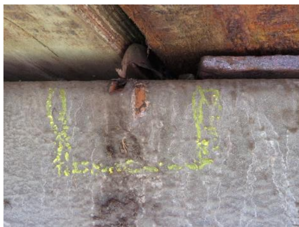
Figure 5.15: Minor deformation at S2-G1
