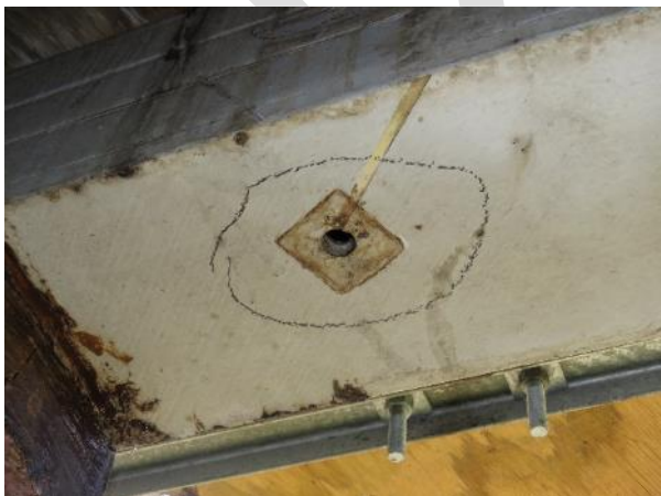
Figure 5.22: View of fibre tear off noted at soffit of girder
