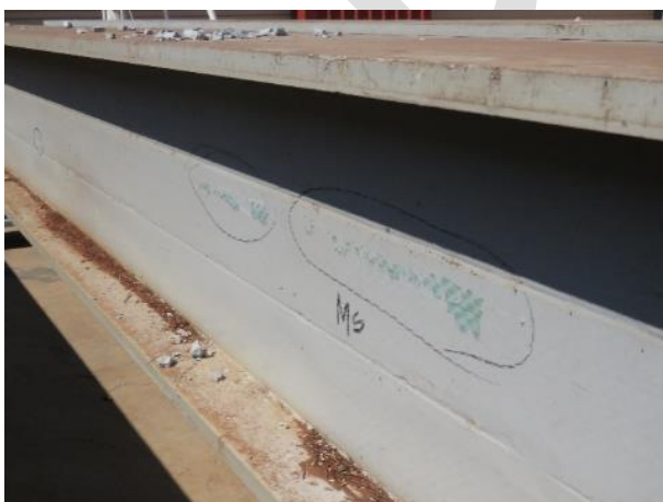
Figure 3.9: Typical blistering and peeling of coating
