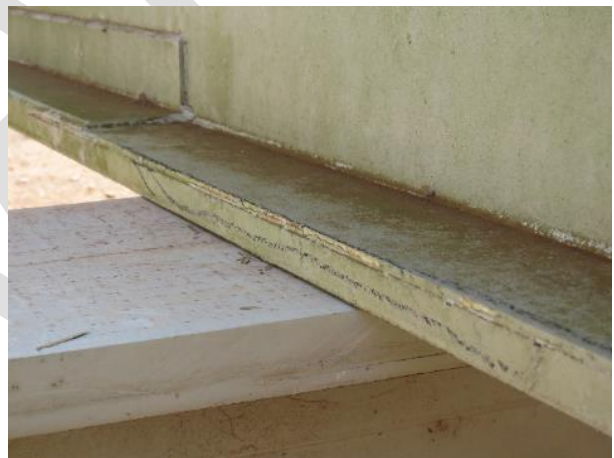
Figure 3.7: Coating deterioration at edge of flange, Girder 1-3
