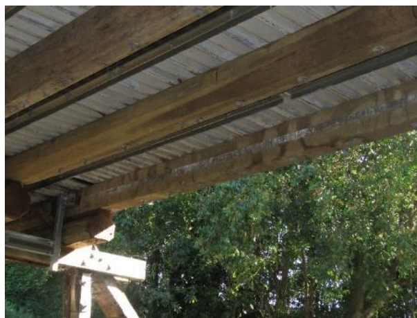
Figure 5.27: Water stains along FRP girder
