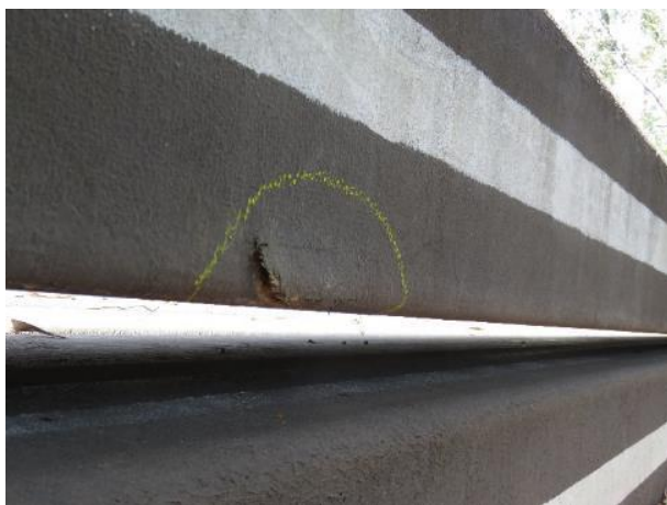
Figure 3.19: Minor tear of the FRP material due to physical impact
