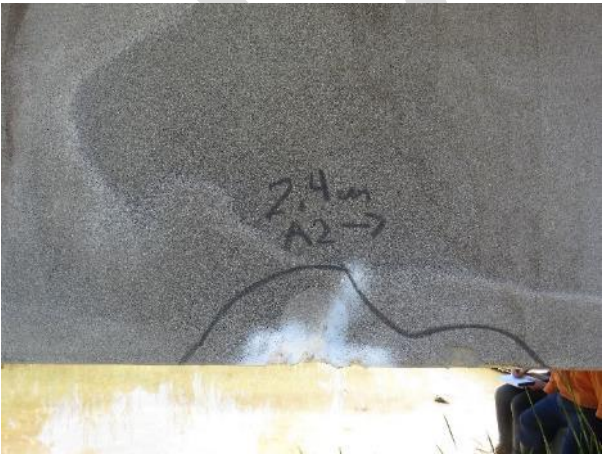
Figure 6.19: Typical spall with exposed fibre along lower edge of girder G3
