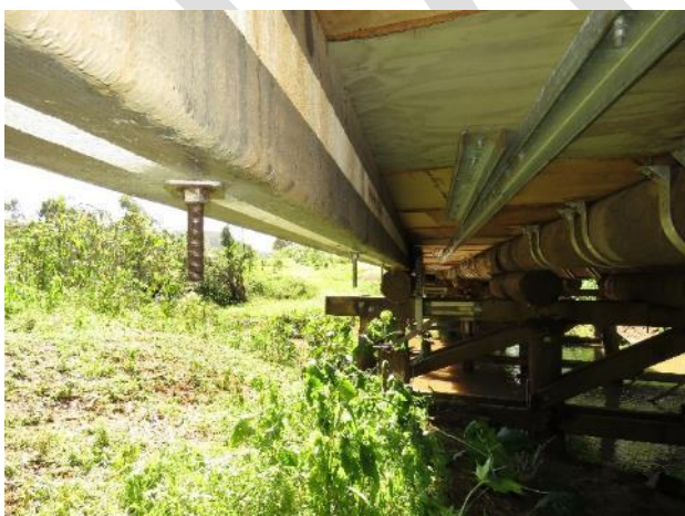
Figure 5.14: Corrosion of bolts at S2-G1
