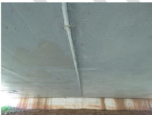
Figure 6.11: Typical water stains on abutment headstocks
