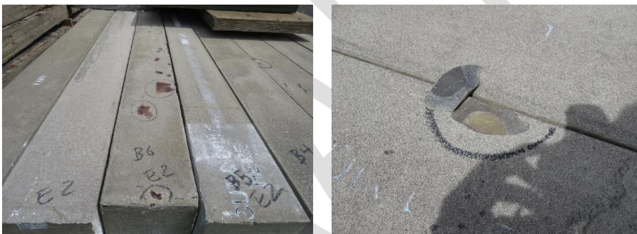
Figure 3.30: Minor damage on coating
