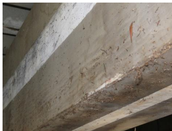
Figure 5.33: View of typical wave shape water stains noted at both faces of FRP girders
