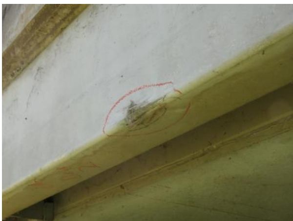
Figure 6.9: Damage on external FRP girder on Span 2
