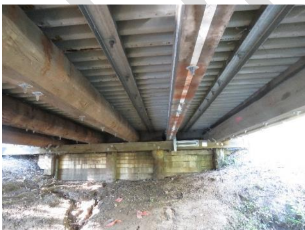
Figure 5.32: Rust-like water stains at the soffit of S1-G2
