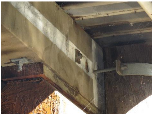
Figure 5.28: Typical minor corrosion of bolts
