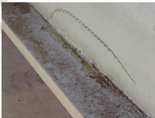
Figure 3.10: Typical peeling of coating noted at the edge of flange
