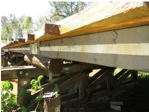
Figure 5.16: Typical water stains on FRP girder
