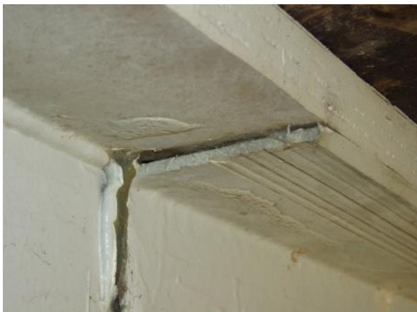
Figure 5.11: Loss of bond between the angle and flange of the girder
