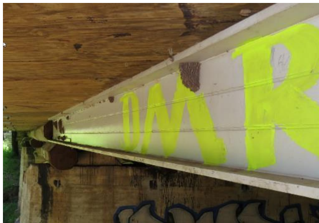
Figure 5.12: Wasp netting on girder's web
