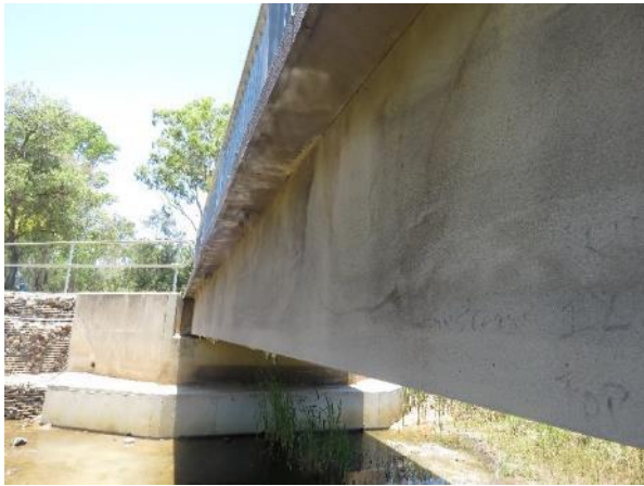
Figure 6.20: Water stains at external face of girder G1
