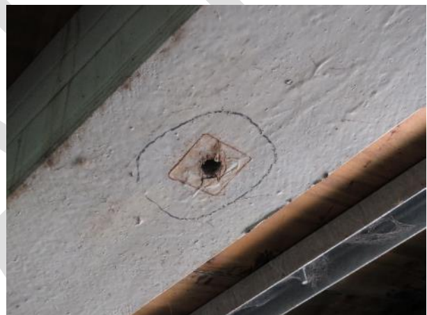
(b) View of a unused hole at the bottom of the girder
