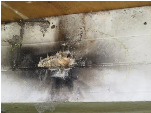
Figure 5.20: View of a burning area noted at right hand side of FRP girder S1G2
