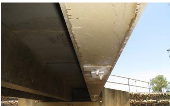
Figure 6.22: Excessive epoxy adhesive at soffit of all girders
