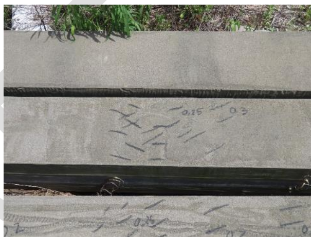
Figure 3.22: Cracking on top of girder 9 at mid-span
