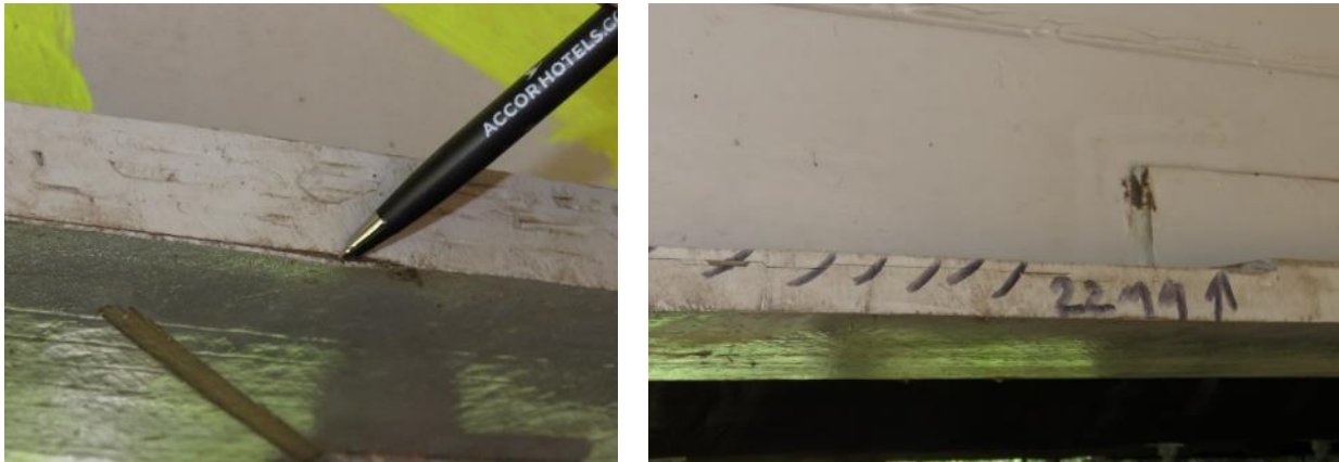
Figure 5.7: Delamination of flange plate at several locations on S1-G1
