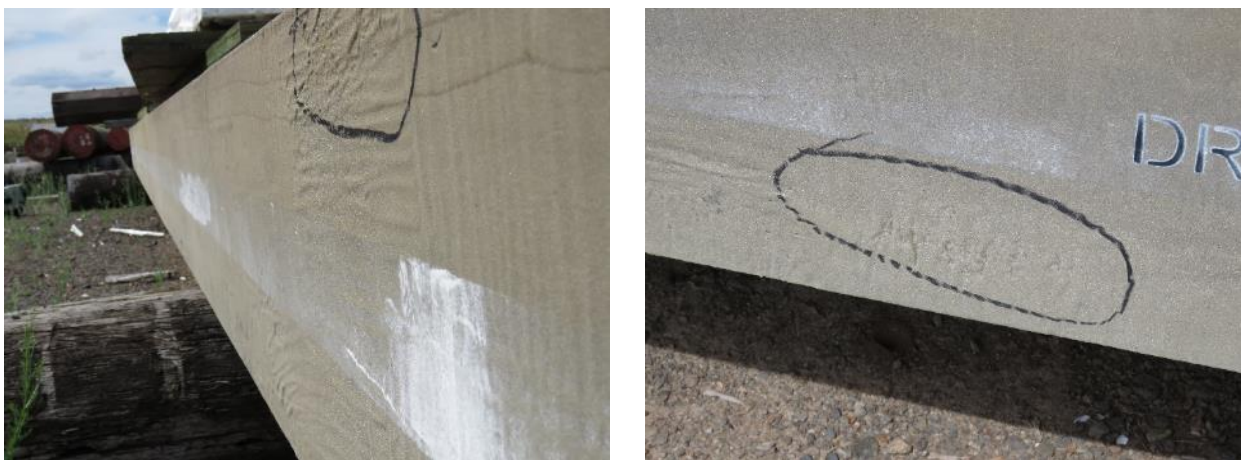
Figure 3.29: Deformation of coating at various locations
