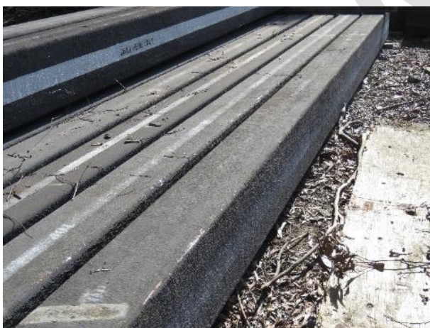
Figure 3.18: Typical loss of coating at girder top edges
