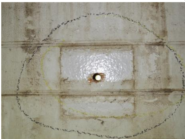
(a) View of a unused hole on the side face of the girder
