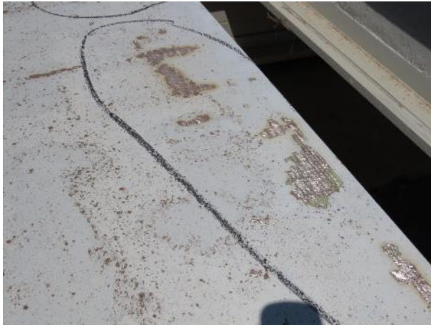
Figure 3.11: Typical peeling of coating at the top of girder G2-6 with fibre exposure
