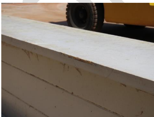
Figure 3.2: Chipping noted at top flange of Girder 1-15
