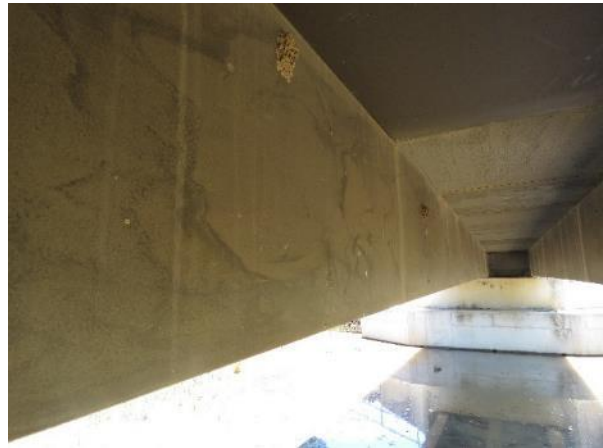
Figure 6.21: Water stains at an internal face of girders
