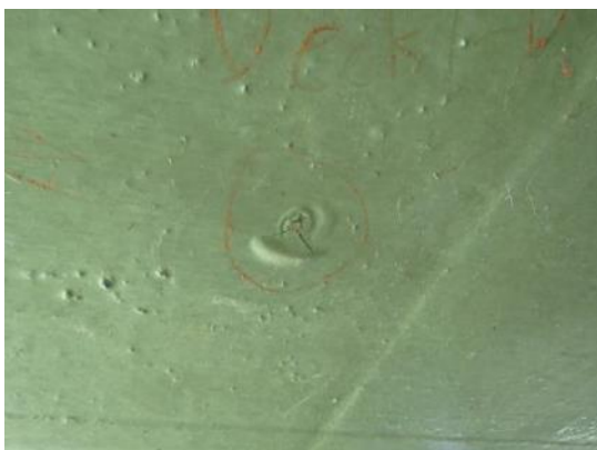
Figure 6.10: Defects on the coating on the soffit of unit 1
