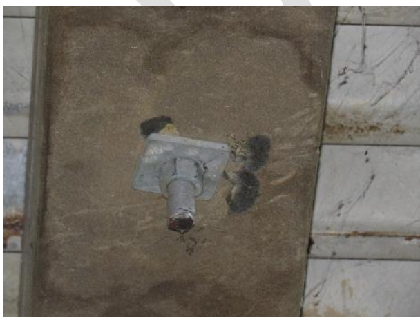
Figure 5.26: Loss of composite and exposed fibres at bolt location
