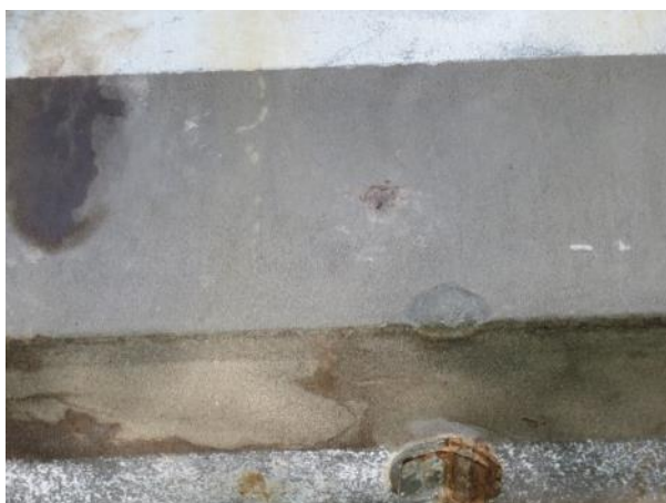
Figure 5.4: View of minor surface deformation due to impact at the RHS end of FRP girder
