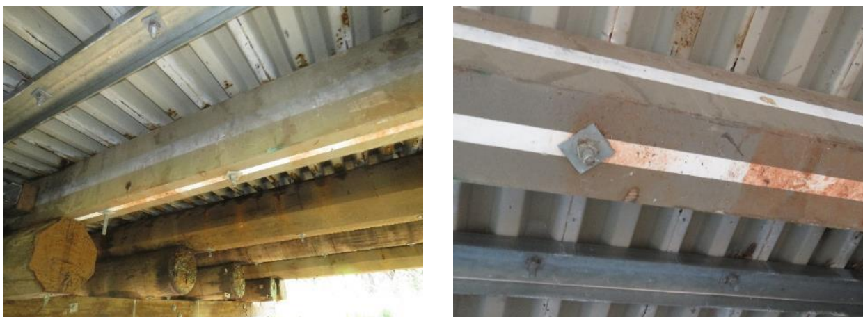
Figure 5.34: Loss of composite and exposed fibres on S3-G2
