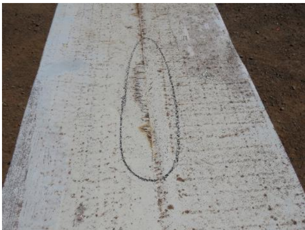
Figure 3.8: Fabrication defect with fibre exposed noted at top and bottom of Girder 1-3
