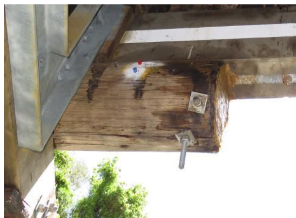
Figure 5.5: Split noted at corbel under end of FRP girder
