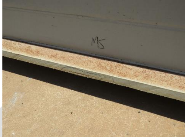
Figure 3.5: Delamination noted at bottom flange of Girder 1-17
