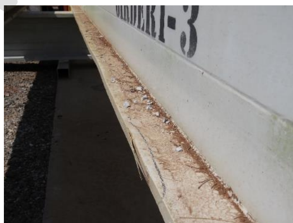
Figure 3.3: Typical chipping noted at bottom flange of Girder 1-3
