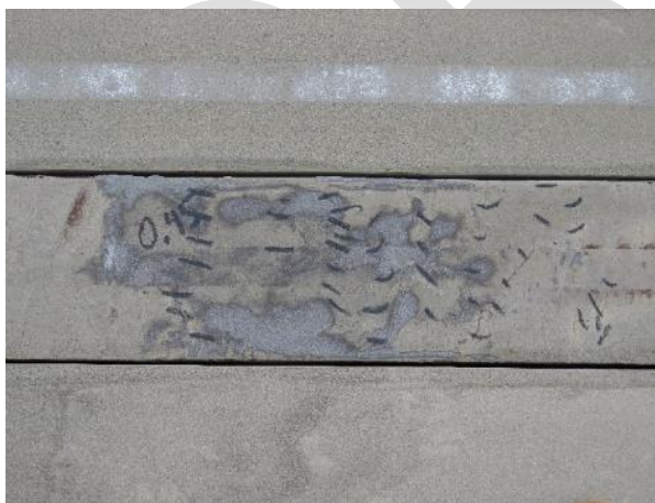
Figure 3.27: Cracking on top of girder 6 at mid-span
