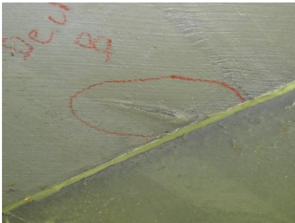
Figure 6.8: Fibre tear and exposed at underside of unit 3 on span 2
