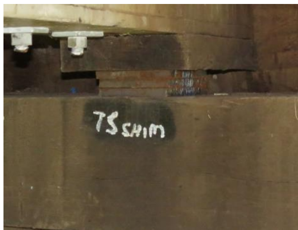
Figure 5.24: View of minor corrosion of steel packers
