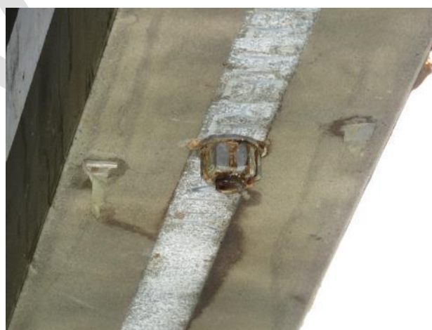
Figure 5.3: Bolt corrosion under FRP girder
