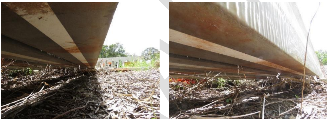
Figure 3.25: Typical rust-type stains at the underside of the girders
