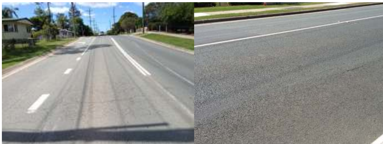
Figure 7.2: Beenleigh Connection Road overview (left) and surface condition (right)
